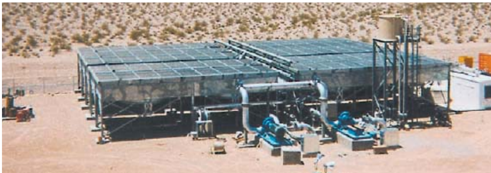
example cooling towers in desert area, Nevada (U.S.A.)
